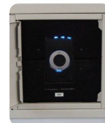
TOP: Wall mounted plate to enable teachers to plug their own USB ABOVE: Classroom self review recording system with locking system
