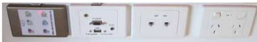
Above: The Control Panel & Wall Plates installed next to the interactive projector
