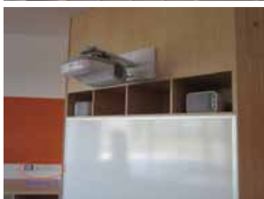
Above: The New ESPSON EB485Wi Interactive Projector installed in the new junior school of Overnewton College
