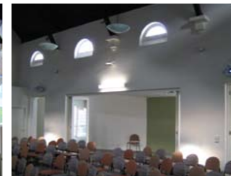
ABOVE: The dual Epson EB-G5200W 4200 ANSI lumen projectors are specially fitted with long throw lenses and discretely mounted on the back wall of the Church.
